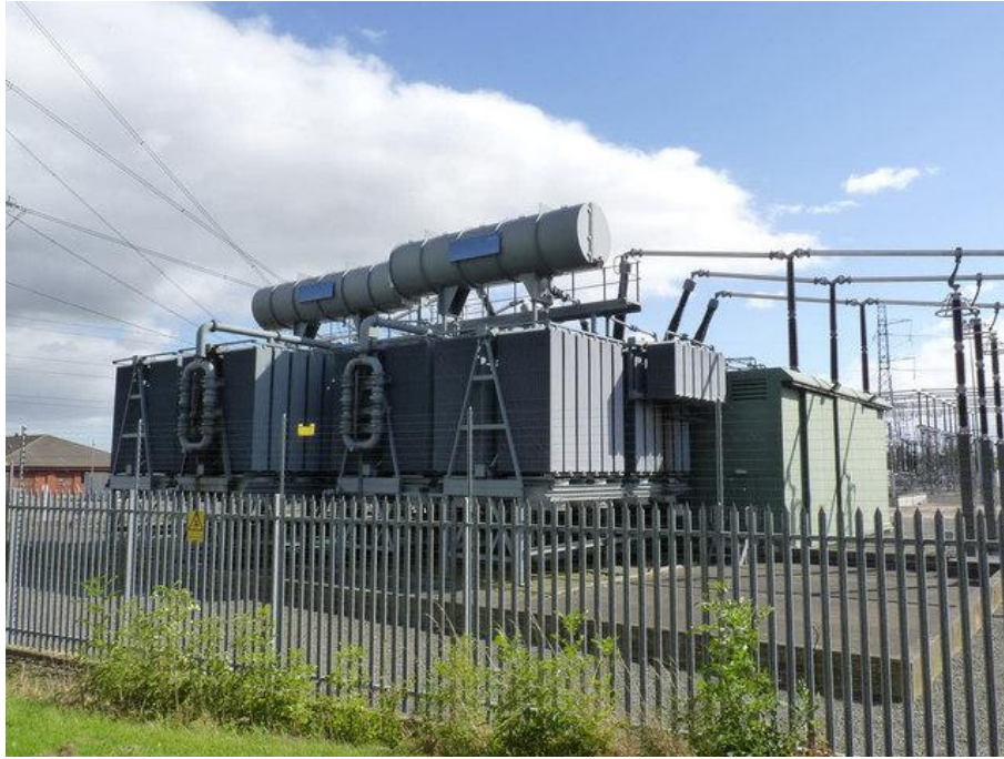
Figure A1.1. Staythorpe switching station, Nottinghamshire: a real outdoor high-voltage AIS installation. The image illustrates repeated steelwork, insulator stacks, conductors and the visually open but extensive character of this form of development. Photograph: [REDACTED], Geograph, CC BY-SA 2.0.
