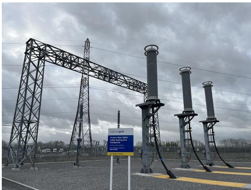
Figure A1.4. National Grid 400 kV cable sealing-end compound at Horsey, associated with the Hinkley connection. The image shows three tall cable terminations, supporting steelwork, conductors, gantry and security enclosure. Image: National Grid.
