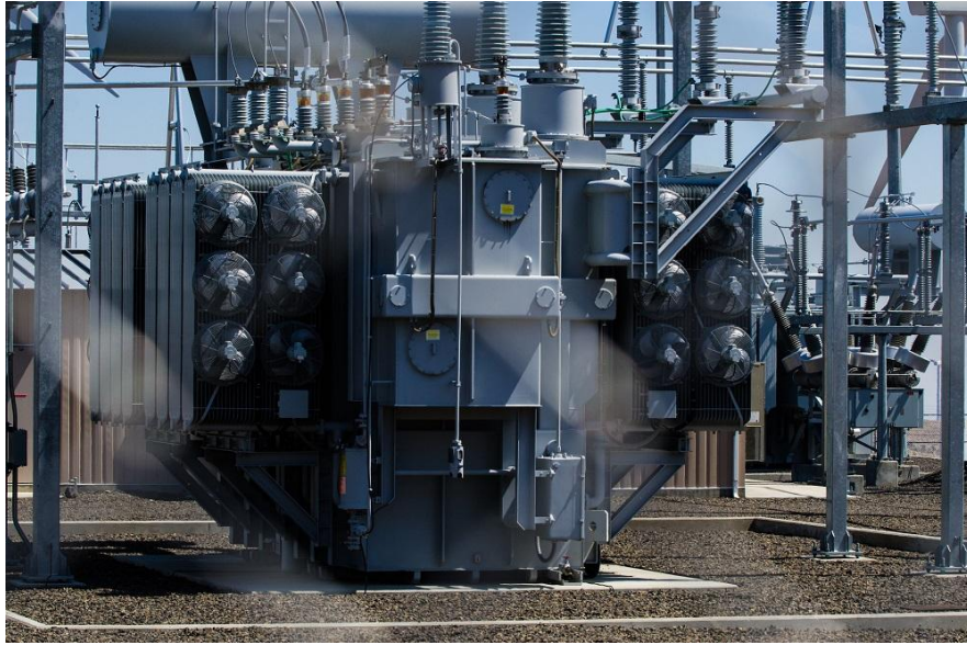
Figure A1.2. Real high-voltage transformer within an outdoor substation. The central tank, cooling radiators, fans, bushings and surrounding busbar equipment demonstrate the solid visual mass that may be obscured by a generic substation outline. This is a real-world comparator, not the proposed East Pye transformer design.
