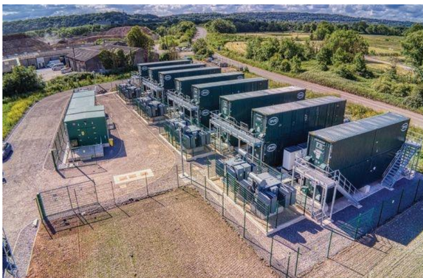
Figure A1.3. Hallen BESS near Bristol: repeated battery modules, platforms and associated transformer equipment. Hallen is a 32 MW/32 MWh facility and is used only to demonstrate equipment form; it is not a scale comparator for East Pye. Image: Wilson Power Solutions.
